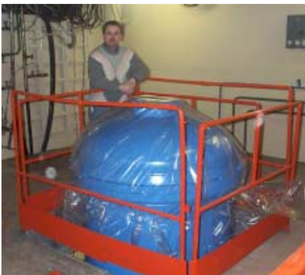
Fig. 4. High voltage power supply tank.
